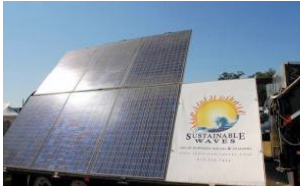
This mobile solar system is providing all the electricity for the main stage at the county fair.
